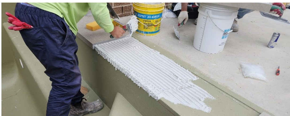
Image 5 - Applying adhesive to both horizontal and vertical areas of substrate using a notched trowel.
